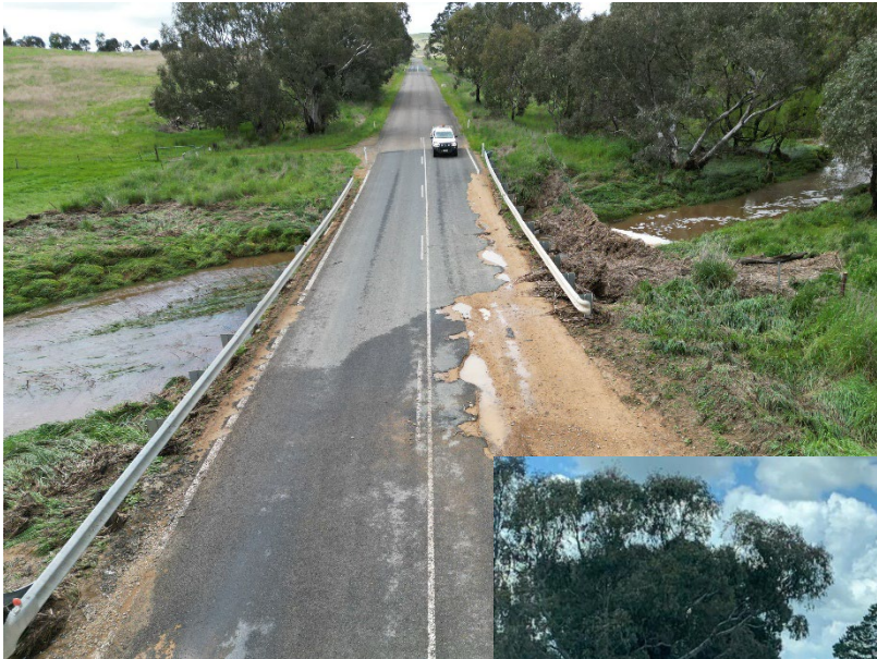
Hardiman Creek floods damage
