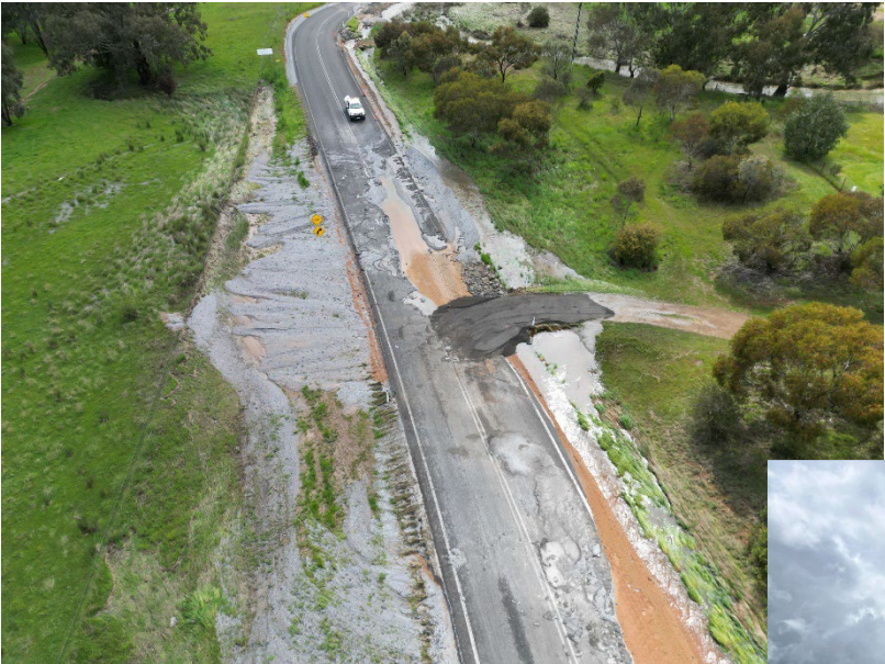
Trucking Yard floods damage
