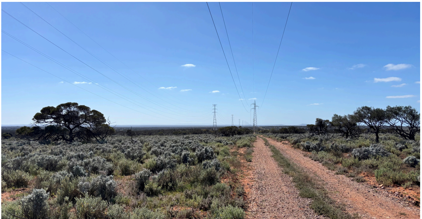
The current Eyre Peninsula Link and Middleback Transmission Lines
